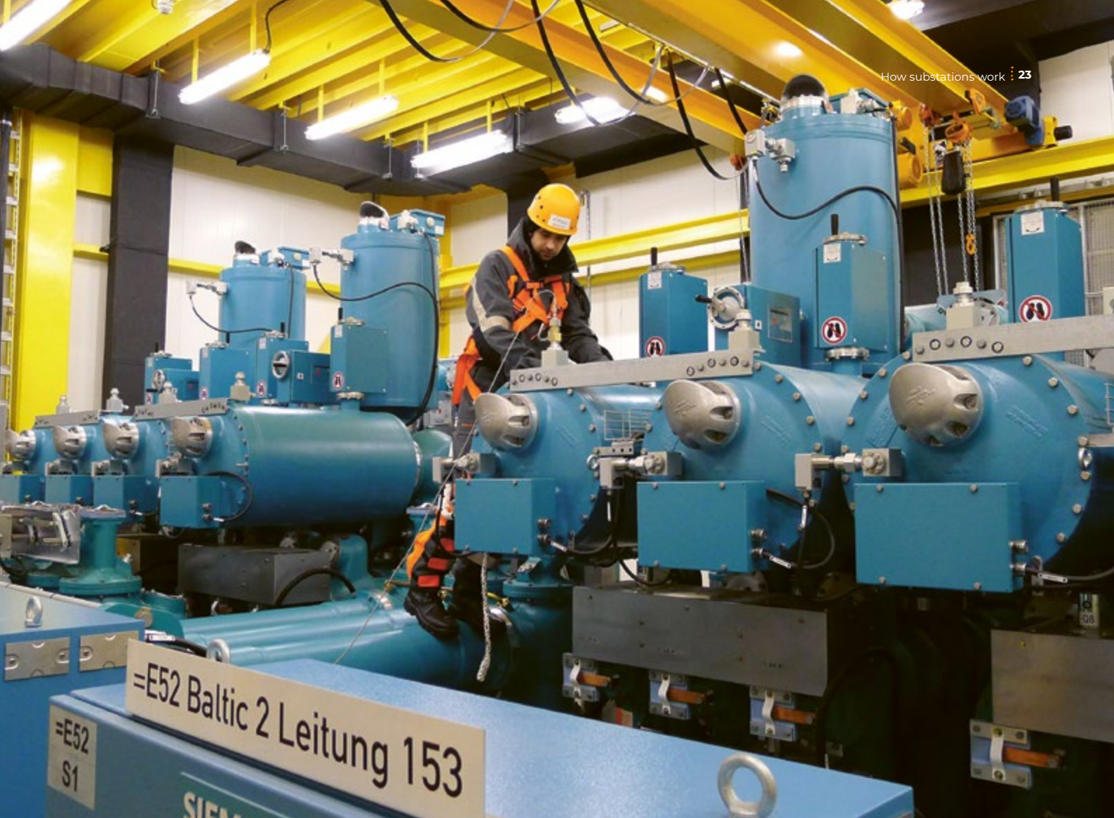
Carrying out inspection work in the switchgear on the platform of the Baltic 1 offshore wind farm.
