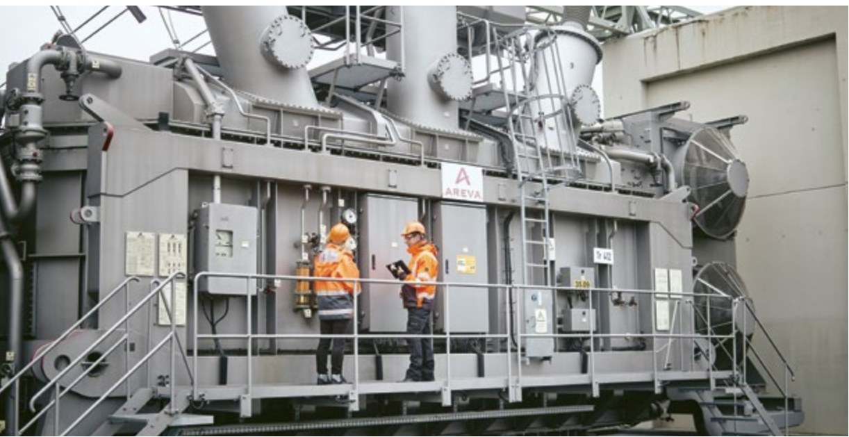
A 50Hertz employee works on a transformer in the Wolmirstedt substation near Magdeburg.
