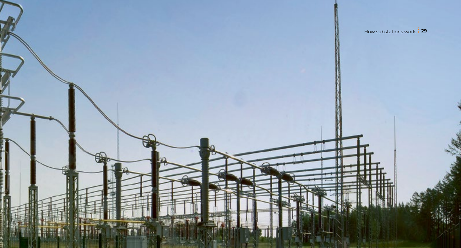
The reactive power compensation system in the Altenfeld substation in Thuringia.
