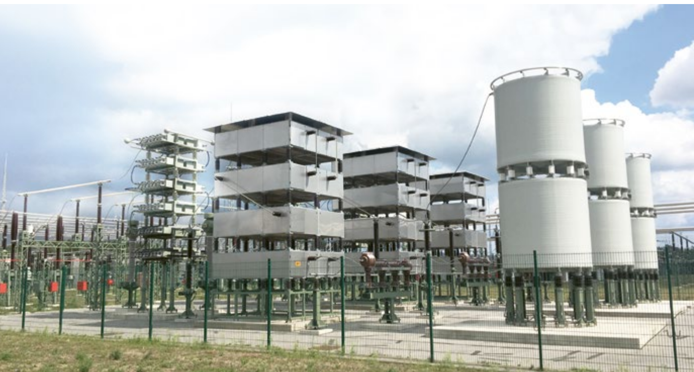
Components of the STATCOM system in the Lubmin substation.
