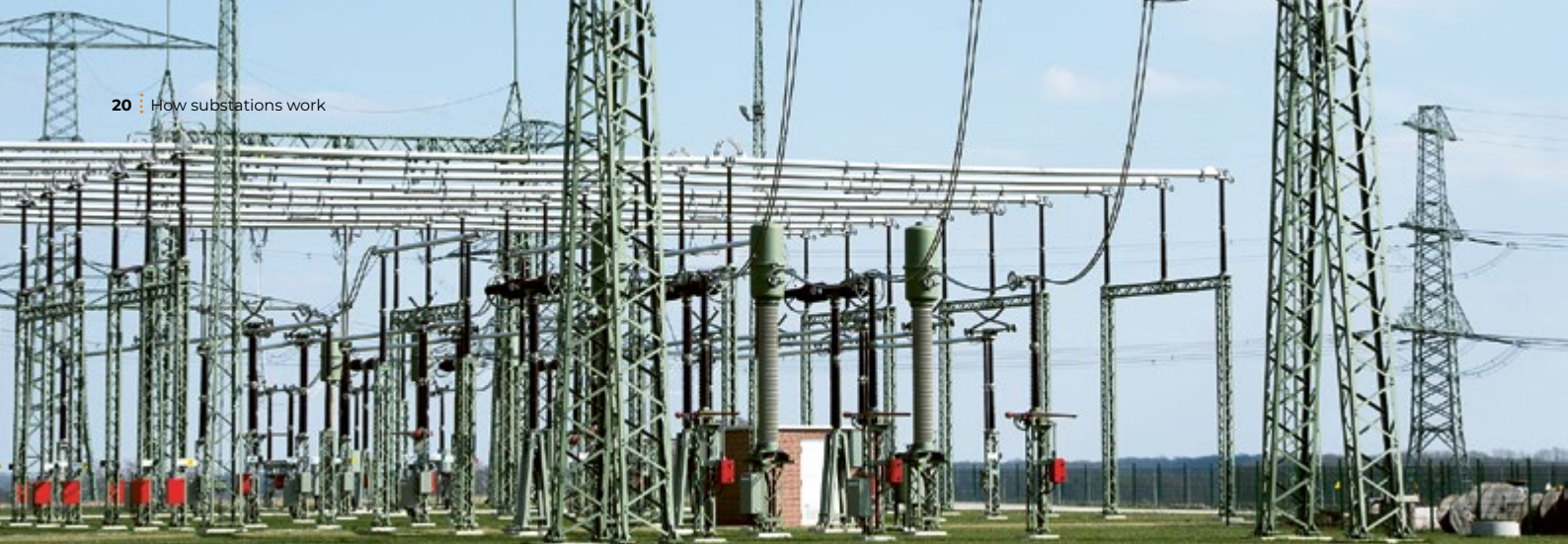
A view inside a 380-kilovolt switchgear in a 50Hertz substation.
